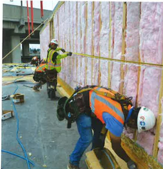
Laying out connections for a Factory_OS unit, Evella Holt, Local 713; Gerardo Garcia, Local 217; and Jose Contreras, Local 22.
