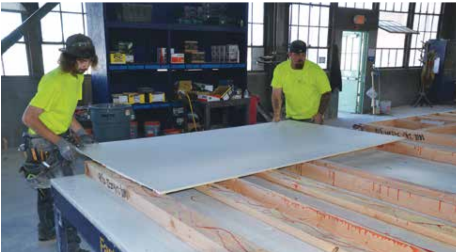
Chance Conner and Caleb Turner prepare to cut drywall for modular units.
