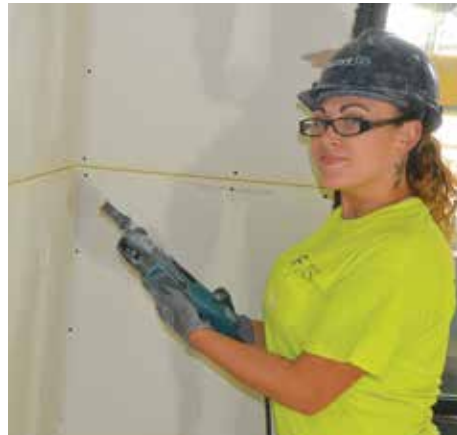
After waiting tables for 15 years, Kimberly Nettles has found a job with good wages, benefits and respect at Factory OS. Here she prepares to install an electrical box in one unit.
