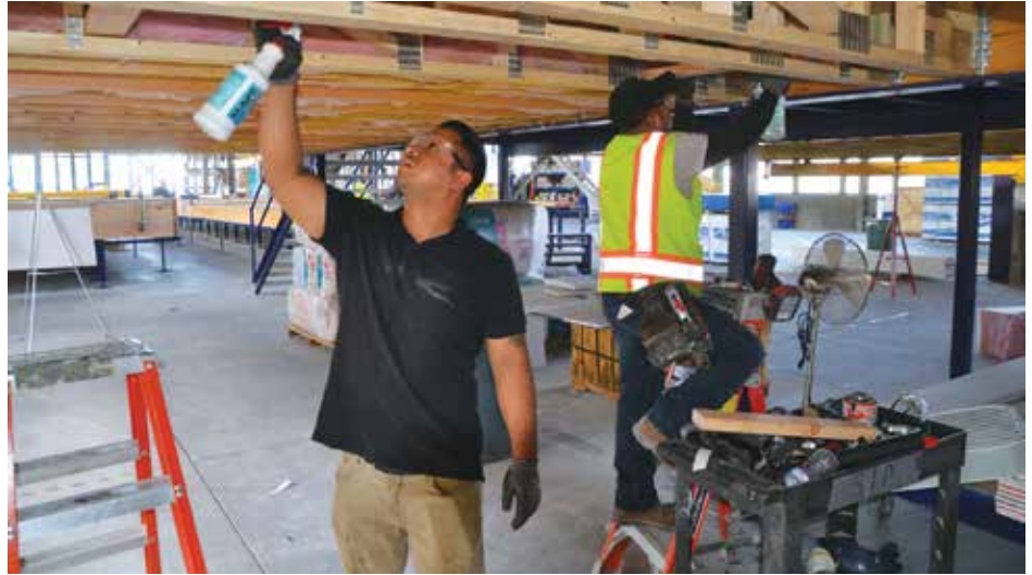
Lead plumber Lissandro Cruz and Carlos Martinez check for leaks under a modular unit.
