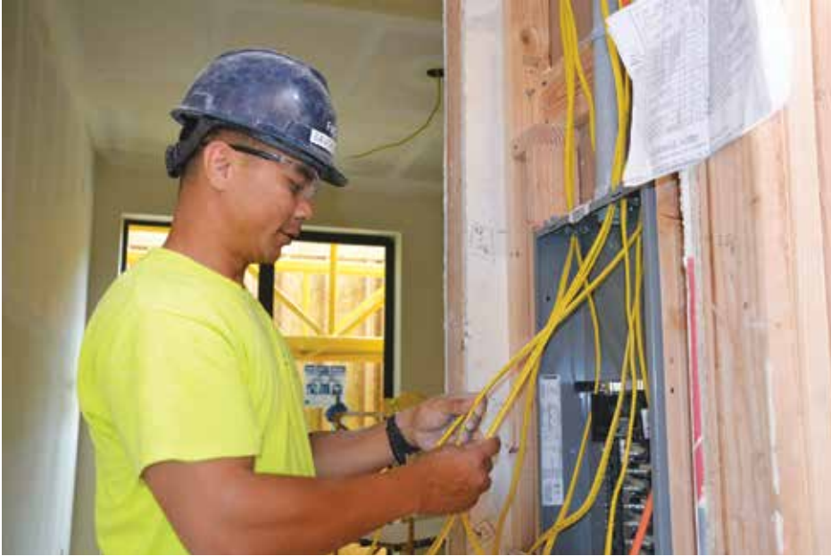
Savony Krouch, a graduate of San Francisco's Delancey Street program for the formerly incarcerated, installs wiring on a modular unit.
