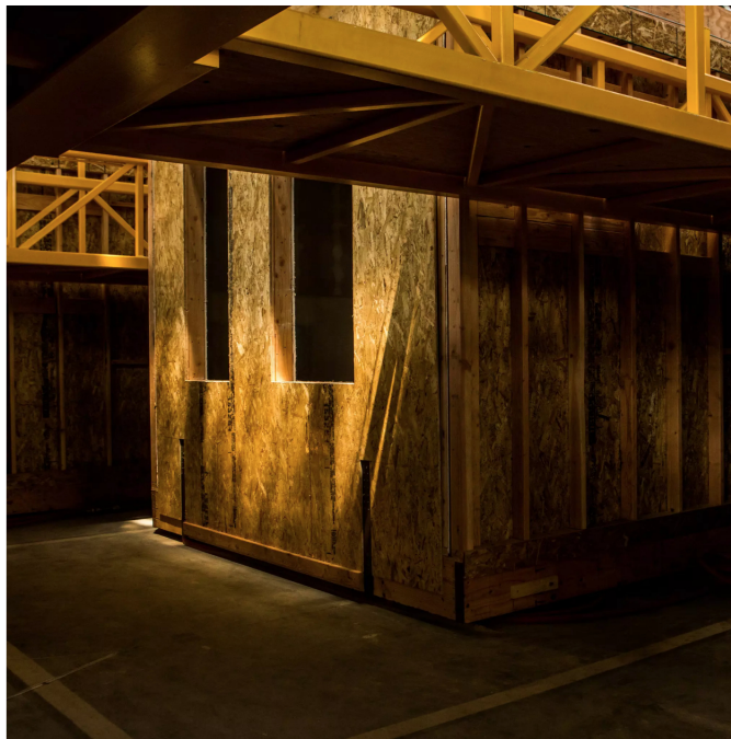
At one set of stations, workers focus on the construction and installation of ceilings for the modular units. Christie Hemm Klok for The New York Times
