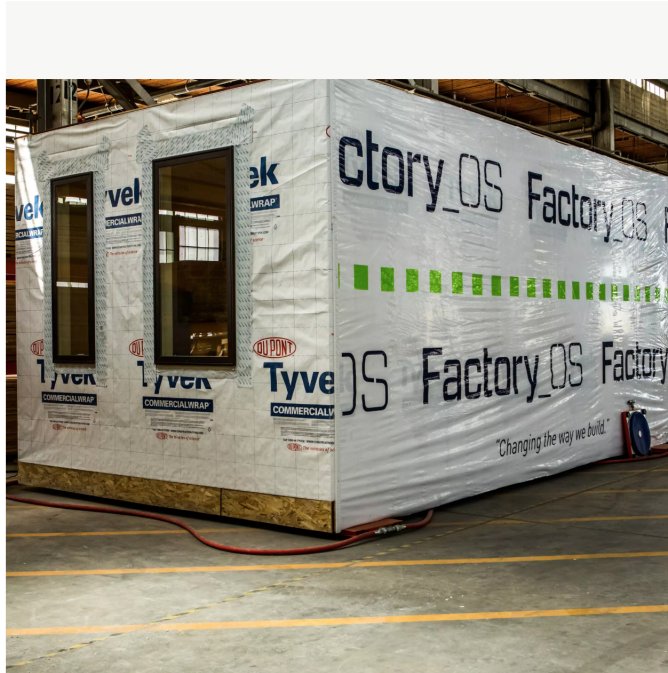
A completed studio unit, ready to be shipped out. The goal at Factory OS is to churn out about 2,000 apartments a year, to be turned into four- and five-story buildings with 80 to 150 units each. Christie Hemm Klok for The New York Times
